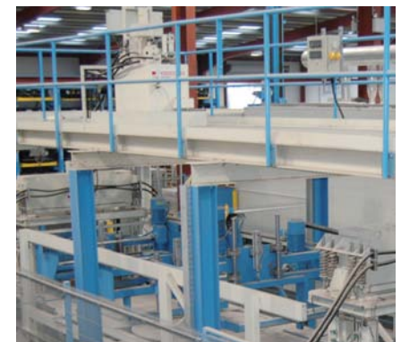
Shot-blasting curling line
