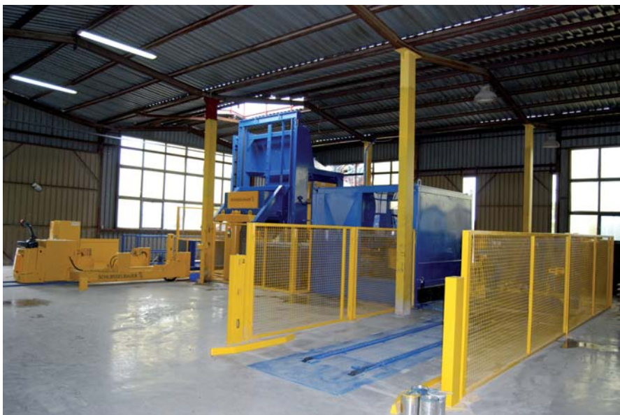
An overview of the new production plant for the production of manhole rings and cones as well as manhole bases at the company ABM Solid.
