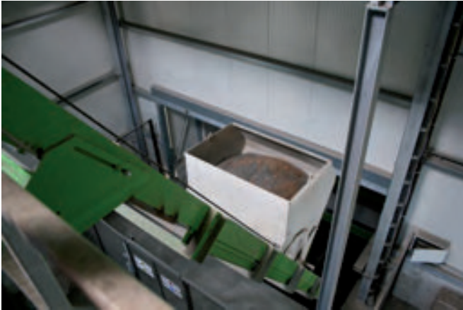
The two mixers are fed via lifts.
