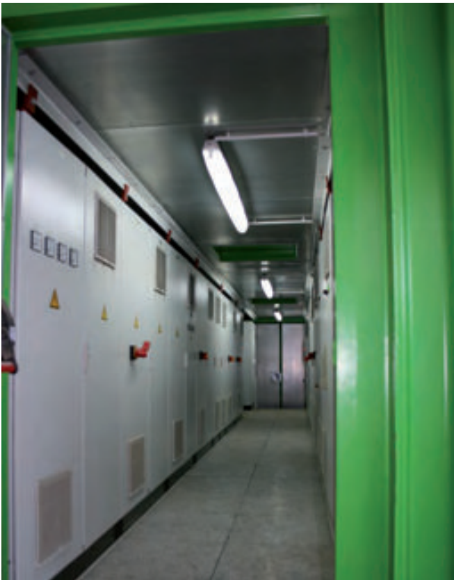
The second powerainer is arranged to the right of the machine room, in which the hydraulic units are located.
