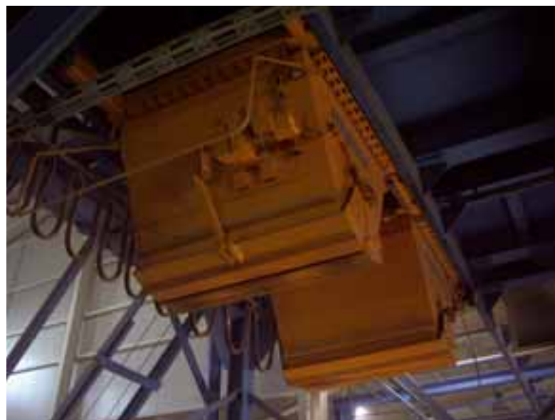
Bucket conveyor system
