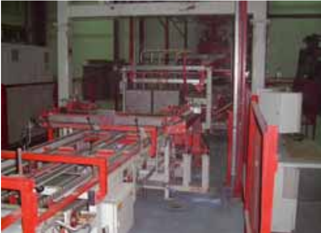
The 1st choice slabs are discharged after refinement via angled transfer units and belt conveyors to the vertical packing station.
