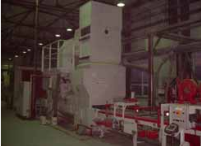
The shot blasting machine is equipped with 2 high-performance turbines, each rated at 15 KW.
