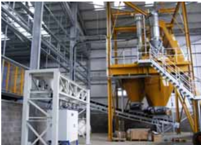
7 tonne batch every 3 minutes are produced by the Haarup 4500 litre mixer. On the left: the Würschum four-colours dosing system
