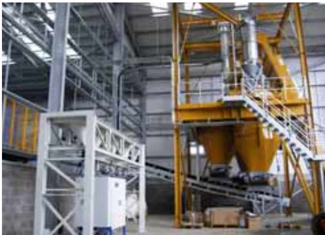
7 tonne batch every 3 minutes are produced by the Haarp 4500 litre mixer. On the left: the Würschum four-colours dosing system
