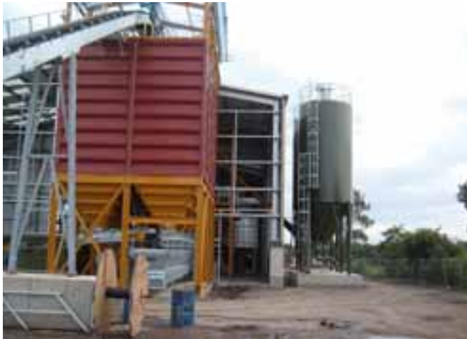
6 x 100tonne storage bins and the 2 x 100 tonne cement silos
