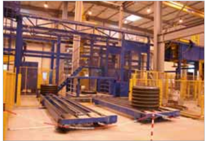
The plant disposes of a fully automatic pallet handling system.
