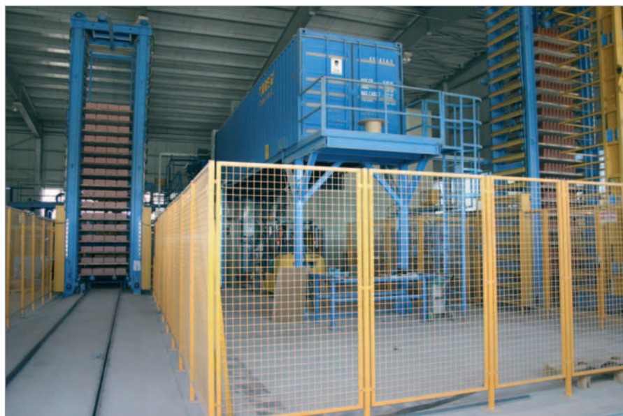
All controllers are pre-installed in the 40' container, which Masa call the 'Powertainer'
