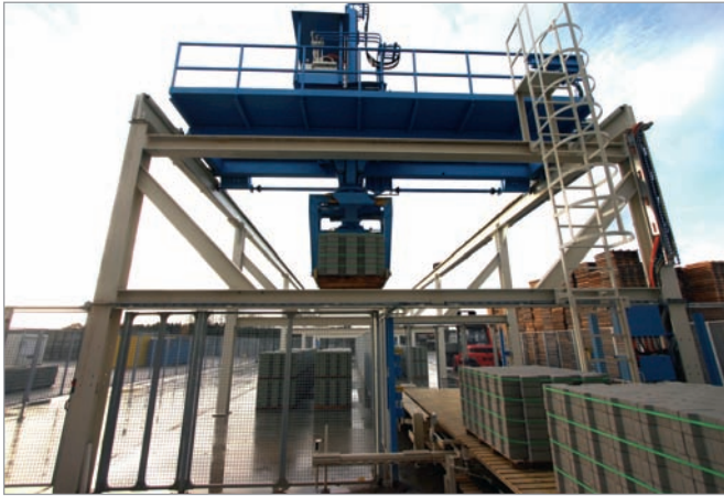
A packet buffer crane was installed outside
