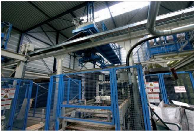
The pallet stacks are fed back to the block manufacturing plant using a sheet stacking crane
