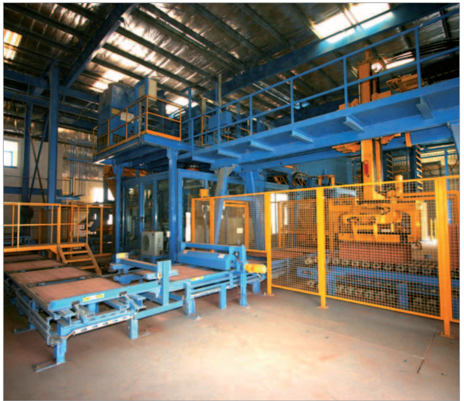
Cross transport of steel pallets and cubing unit with slat conveyor
