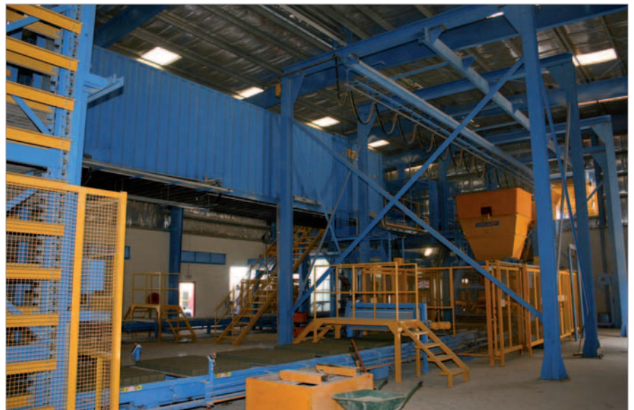
Product transport at the wet end and switch cabinet container
