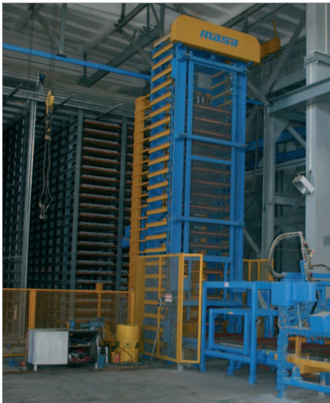
The H&S shelving units were supplied in the form of a closed system with recirculating air equipment
