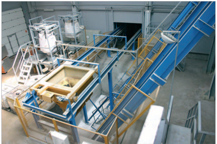
The aggregates are weighed and filled into the mixer elevators from the charging scale
